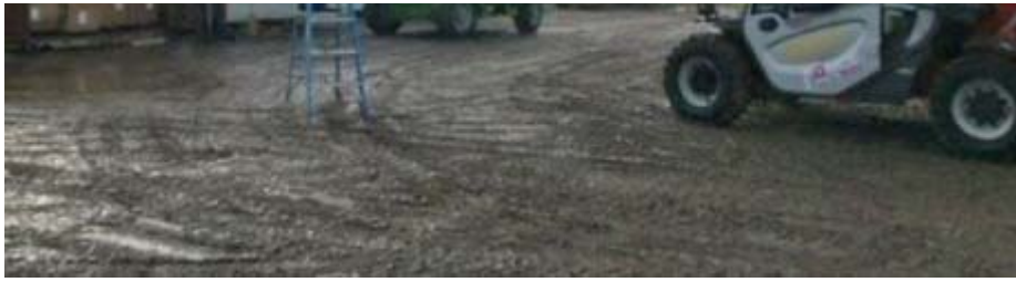
PHOTO Construction is underway on the glasshouse in the Hunter Valley region of NSW.
